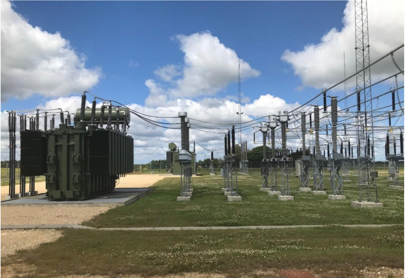
130/150kV transformerstation - European Energy
